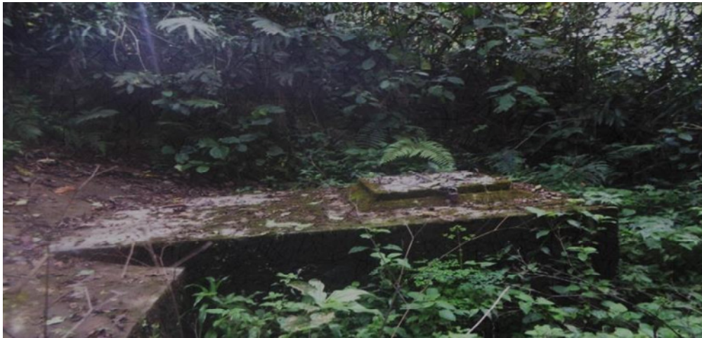
Figure 1: Nguvinkei II Water Supply collection tank
